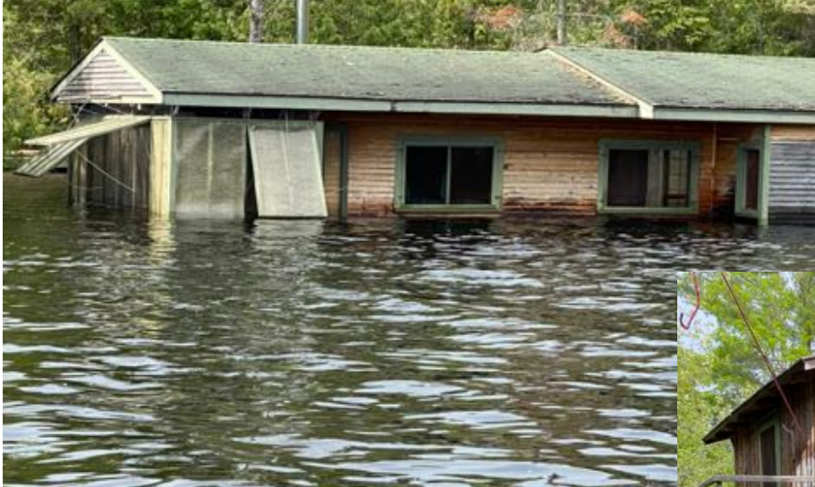
Cedarbark House - water lapped into the windows
