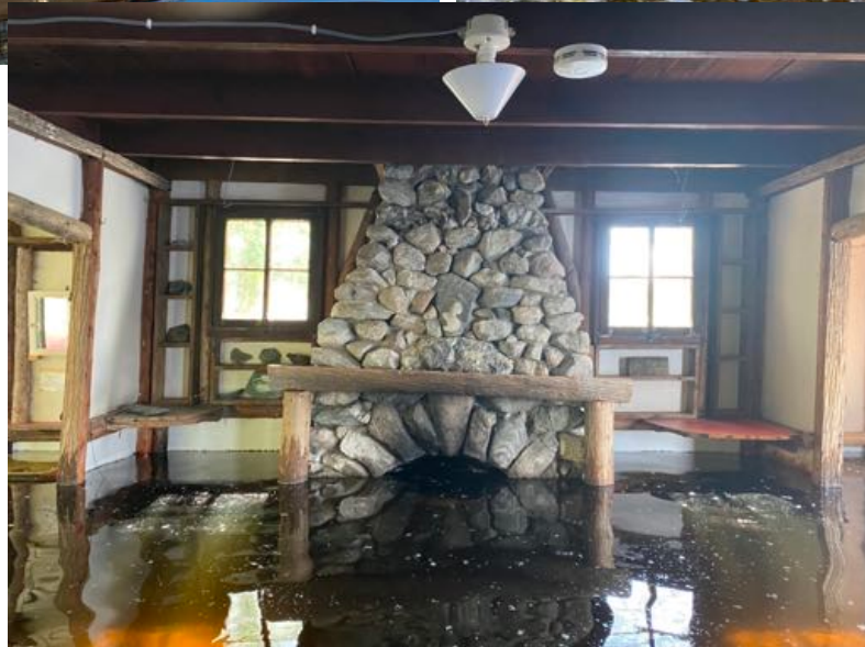
Cedarbark House firebox full of water
